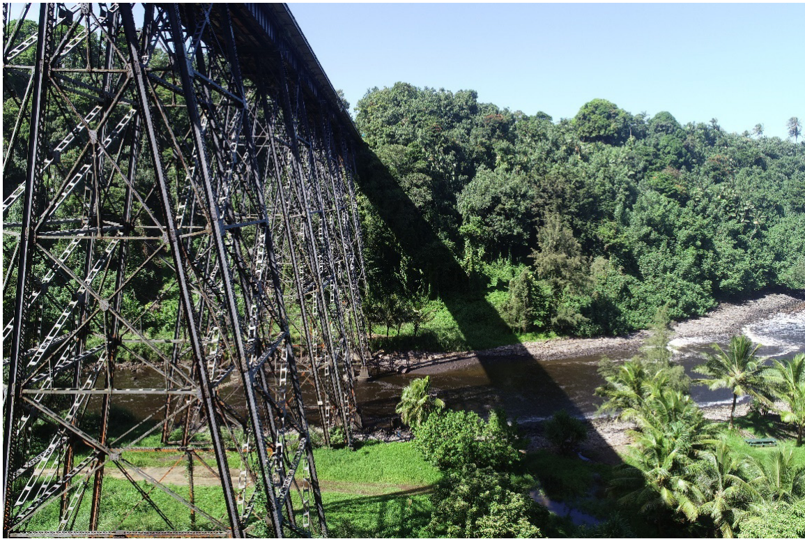
Figure 2. Example of Bridge Trusses where Workers Traditionally Work at Height (Image Courtesy: FHWA Western Federal Lands Highway Division)
