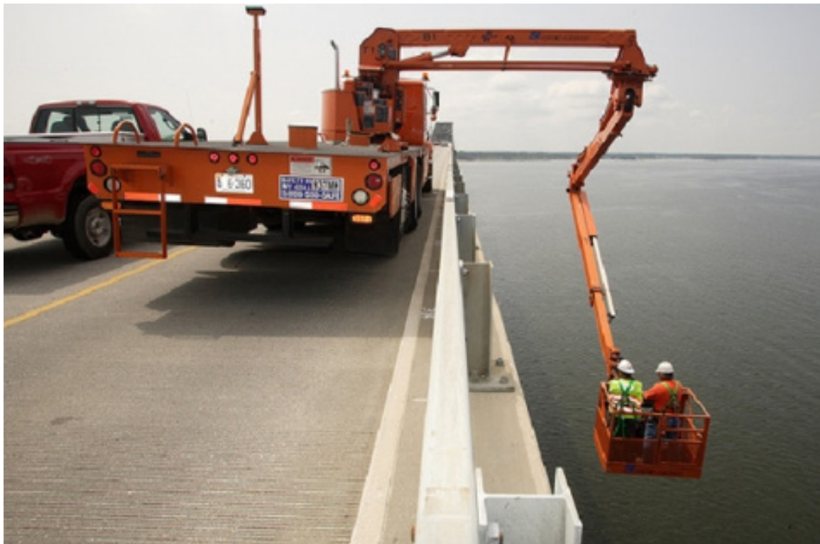
Figure 3. Example of Workers Conducting Bridge Maintenance from a Snooper Carriage (Reproduced from (Chen, 2014)) 7
