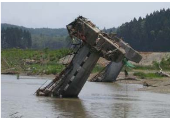
Figure 18. Damaged piers of the JR Rail Viaduct at the Tsuya River.
