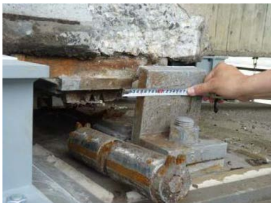
Figure 19. Ejected roller bearing and longitudinal movement at a pier of the Yuriage Bridge.
