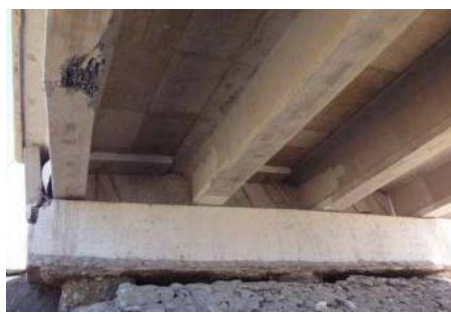
Figure 15. Girder bottom flange damage in the Chada Bridge due to the Maule Earthquake.
