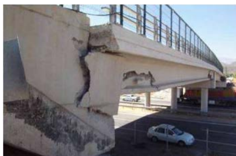
Figure 14. Abutment wall shear failure in the Chada Bridge due to the Maule Earthquake.
