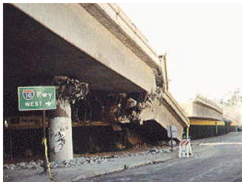
Figure 10. Collapsed bridge section of westbound Santa Monica Freeway due to the Northridge Earthquake.
