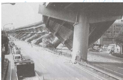
Figure 12. Failure of the Piltz Bridge due to the Hyogoken Nanbu Earthquake.
