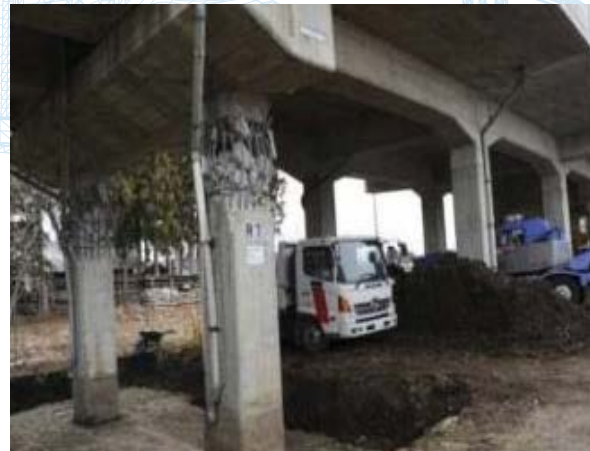
Figure 17. Damaged columns in the Nakasone Viaduct.
