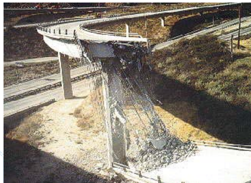
Figure 11. Collapsed connector structure at the Golden State Freeway due to the Northridge Earthquake.
