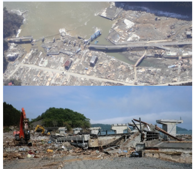
FIGURE 1. UTATSU OHASHI BRIDGE LOCATED ALONG JAPAN'S NORTHEAST SHORE WAS SEVERELY DAMAGED, INCLUDING SUPERSTRUCTURES WASHED OUT BY THE TSUNAMI WAVE FROM THE 2011 EARTHQUAKE. SOURCE: FHWA/PWRI 4
