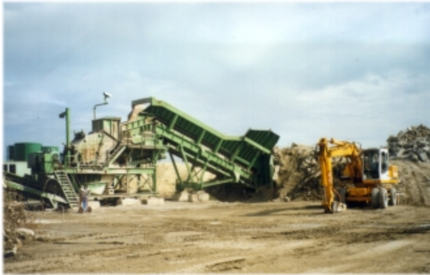
Figure 25. The concrete crushing Jean LeFebvre C&D waste recycling plant in France.
