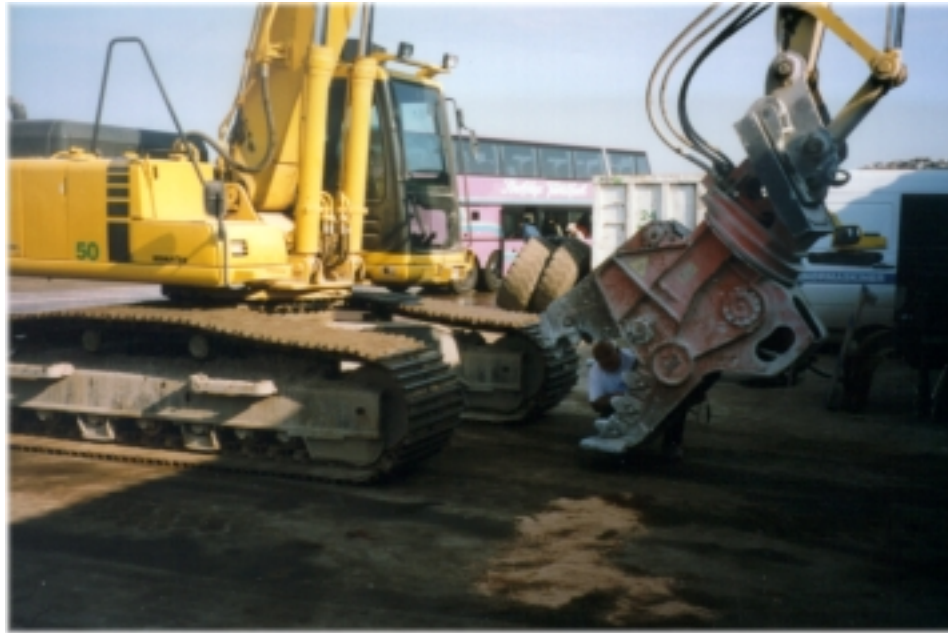
Figure 11. Concrete jaw crusher at the RGS 90 A/S materials processing plant in Denmark.
